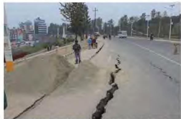
Photo. 6 Valley fill collapse in the Kathmandu airport road.
