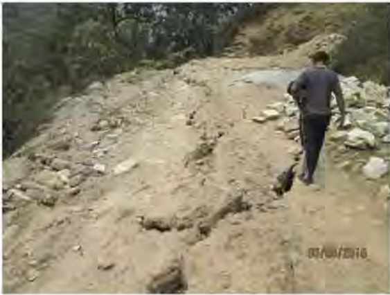
Photo. 7 Failure in Cut-and-fill part of rural road (Photo: Prem Khatri)
