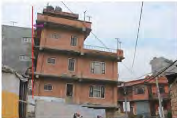
Photo. 8 Land subsidence and tilting of house due to liquefaction of lower strata
